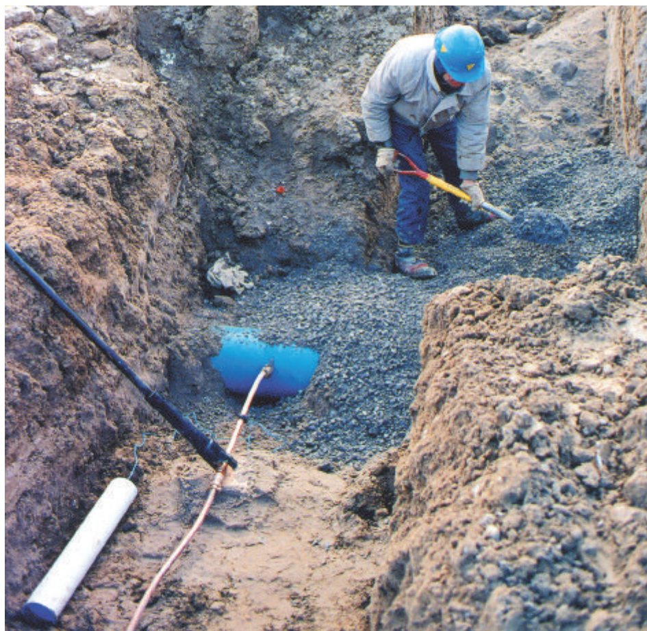
Backfilling of an underground water installation, showing the main, service, anode and curb stop.
