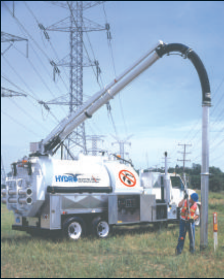
Vacuum excavation is used in some locations for water works installations. A Vactor® HXX™ HydroExcavator is shown. Photos: Vactor Manufacturing, a subsidiary of Federal Signal Corporation.
